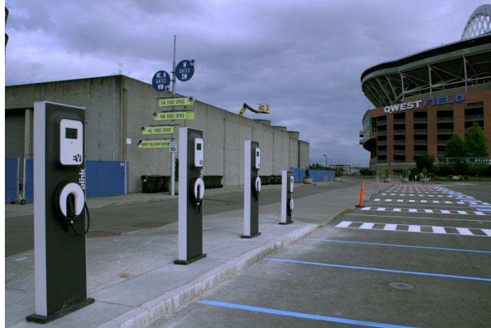
Figure 10. Typical alternating current Level 2 public charging station.
